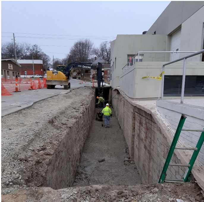
Sidewalk removal and traffic control along the North side of Jefferson Street next to J&S
