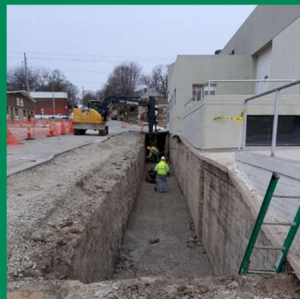
Sidewalk removal and traffic control along the North side of Jefferson Street next to J&S
