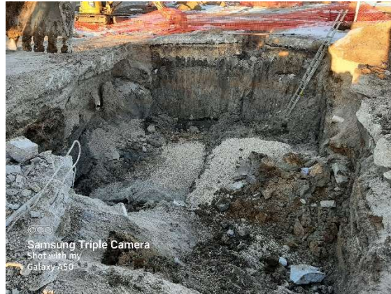
Boring pit preparation in parking lot for water main and sanitary sewer.
